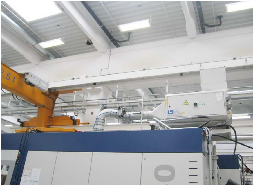
Figure 8 Shut-off valve for air, extinguishing nozzle and flow sensor
